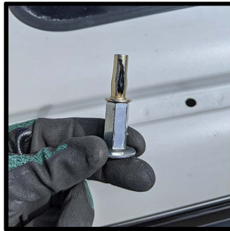
Be sure to clean any shavings away that fell thru while drilling Then apply a thin layer of silicon before inserting the plusnuts
